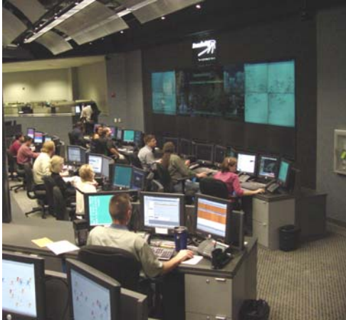
Network Operations Center (NOC) Austin, TX
